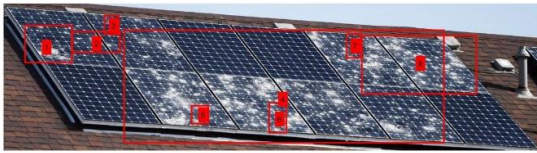
Fig. 17. Detected Cracked PV Panels (see [12]; original image adapted from [15])
